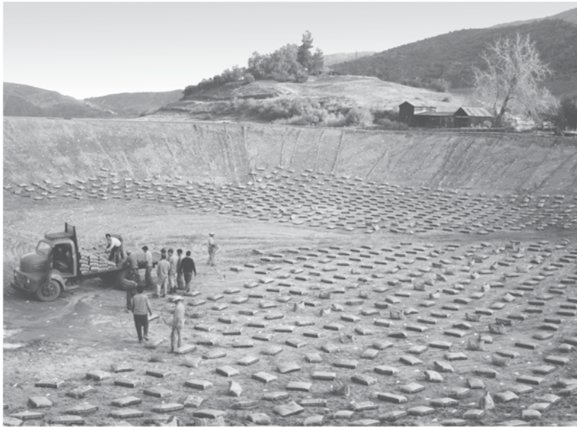
In 1962, the economical method for lining reservoirs was soil cement. Bags of cement were mixed into the soil at the Jameson-Teague property in Horsethief Canyon.
