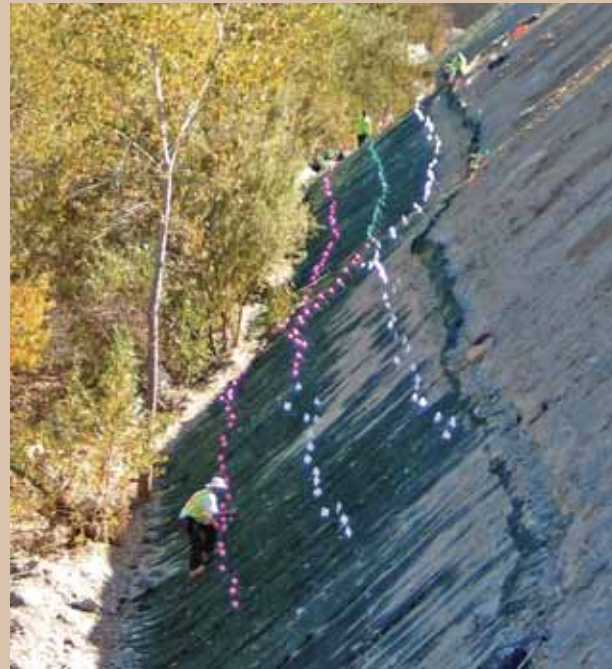
A woven, high performance mat was installed and interplanted with vegetation to strengthen the channel bank.
